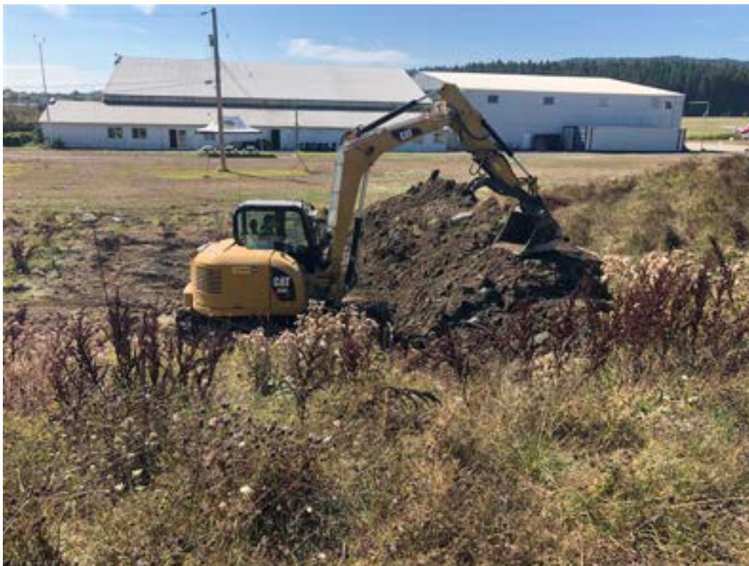
Photo 16: View looking south at Contractor using existing stockpiles to create berm for containment cell in the stockpile management area. Berms were covered with polyethylene liner to segregate from other stockpiled material.
