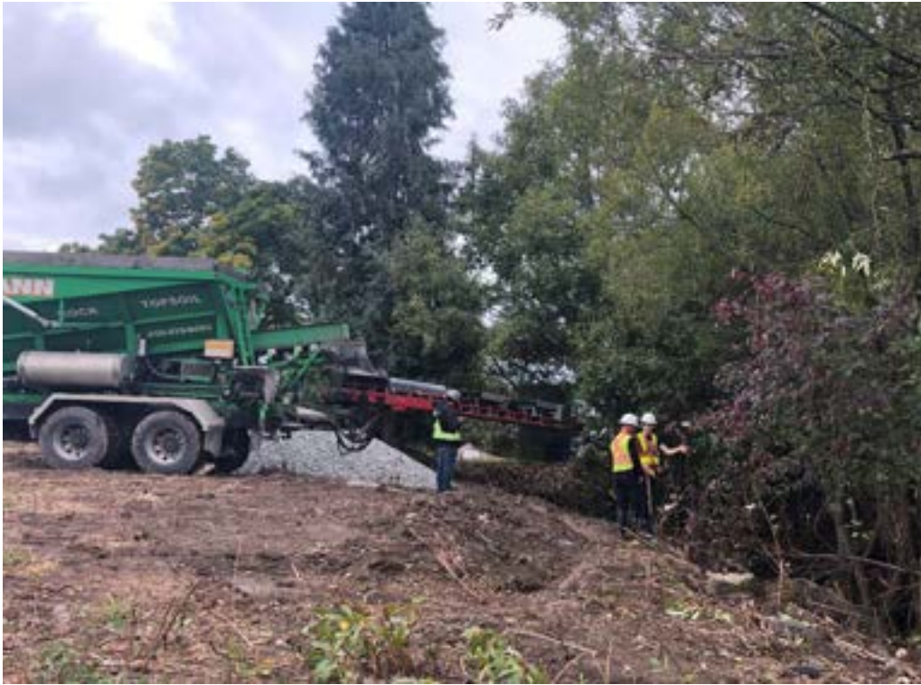
Photo 21: Slinger truck placing backfill in Reach 1C where excavator access was limited.
