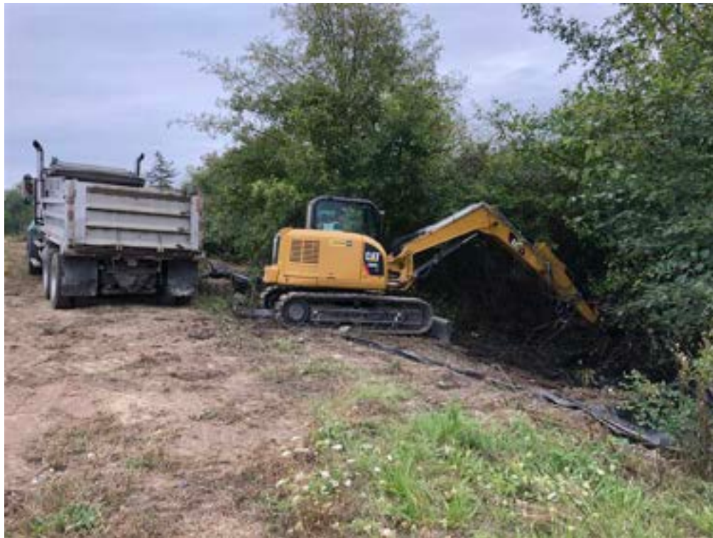
Photo 13: View of remedial excavation in Reach 1A, looking east. Excavated sediment was placed in dump truck and transported to the stockpile area.
