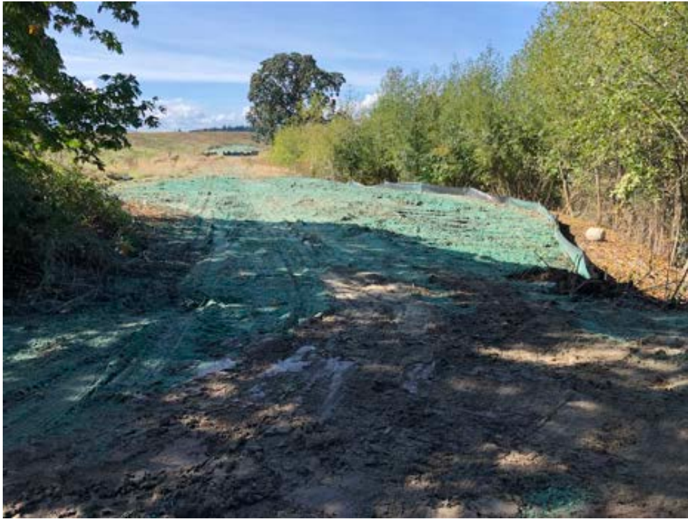
Photo 27: View looking west at the southern side of upper Reach 1C post-hydroseed and silt fence installation.
