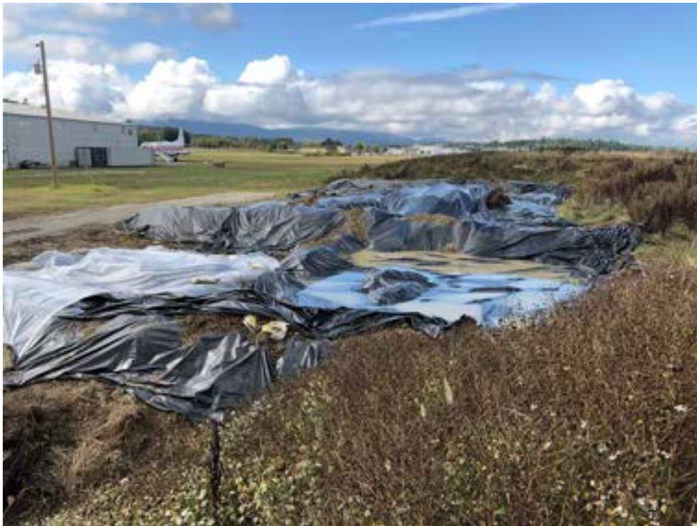
Photo 17: View of excavated sediment in containment cells lined and covered with polyethylene liner, looking west.
