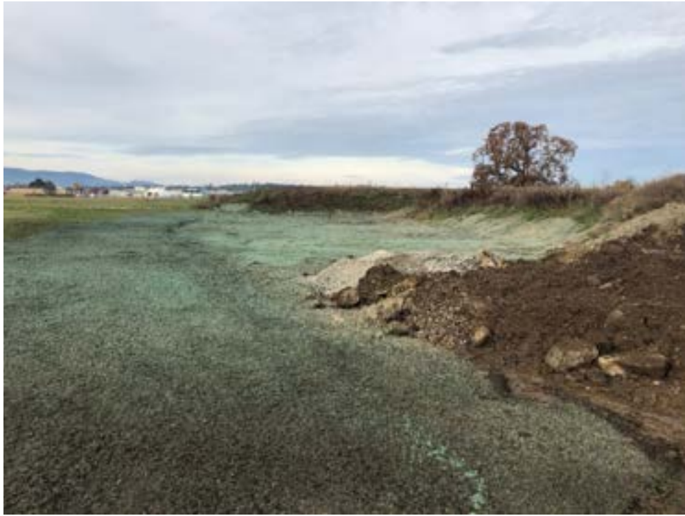
Photo 25: View looking west at the stockpile management area after stockpile removal, remaining VAA material is seen on the right.
