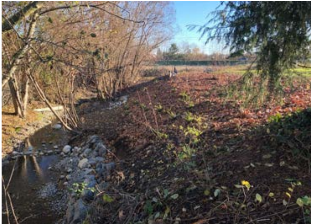
Photo 26: View looking downstream (east) along lower Reach 1C. Western sword fern plantings with leaf mulch can be seen along the stream edge and bank. VAA installed retaining wall can also be seen on the lower left.
