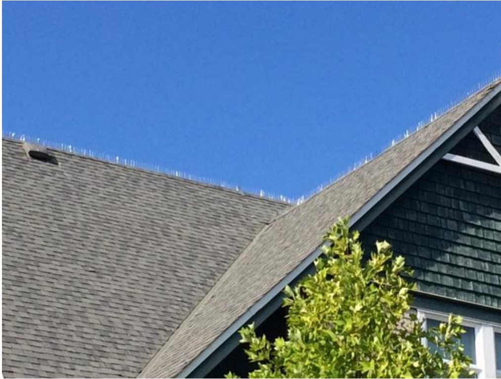
Appendix Figure 19. An effective use of spikes on the peak of a roof.
