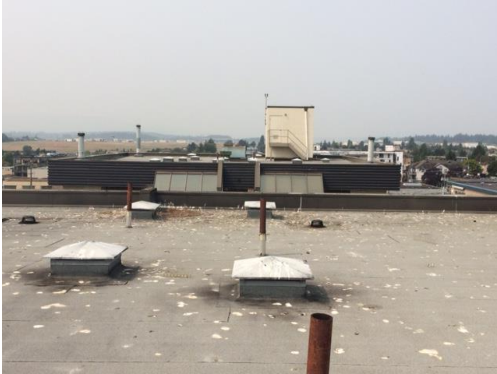
Appendix Figure 29. Lots of feces buildup on a flat roof without gull deterrents, e.g. spikes.
