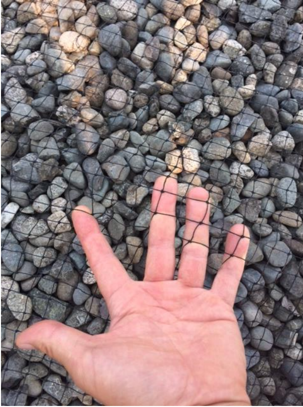
Appendix Figure 21. This netting has been installed on the Sidney Hotel and Spa to prevent gulls from picking up the rocks and dropping them on glass surfaces. It does not deter nesting though.
