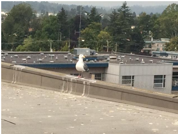
Appendix Figure 26. An example of a gull perching on a portion of a roof edge where the spikes have been knocked out of place.
