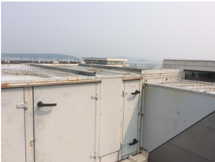
Appendix Figure 24. It is important to place the spikes on all infrastructures on a roof; otherwise the gulls will use the accessible perches.
