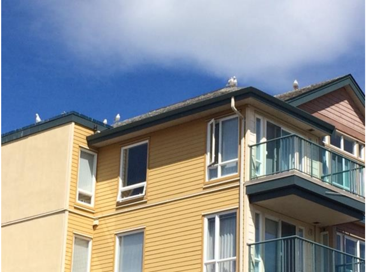
Appendix Figure 7. A close-up of the building in need of exclusionary spikes or wires.
