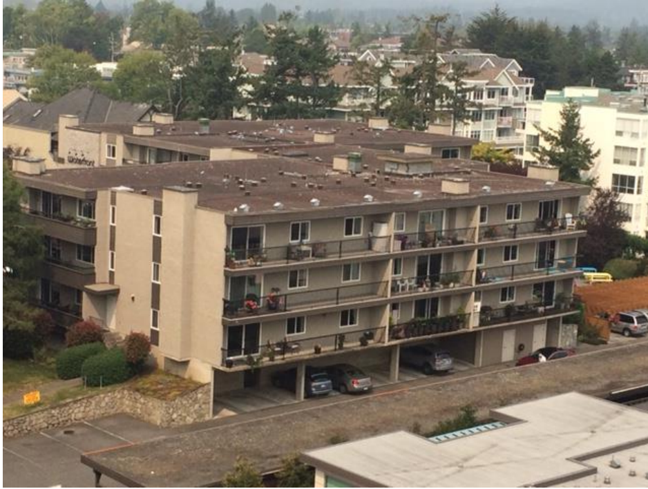
Appendix Figure 31. A roof without deterrents like this one provides a perfect roosting and nesting site for glaucous-winged gulls.
