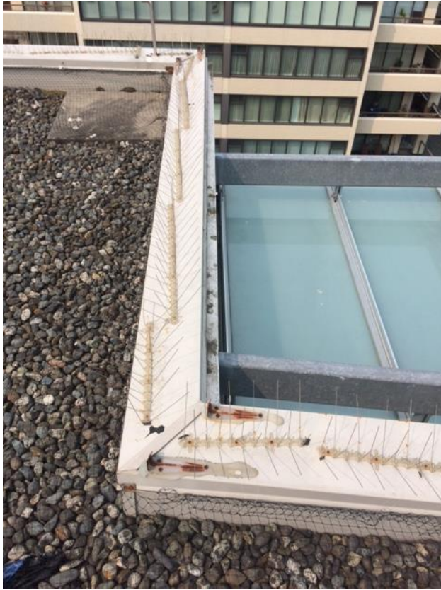
Appendix Figure 25. The magnets holding these spikes are not strong and thus, the gulls can knock them out of place; use of some sort of bonding glue is advised for total, long-lasting effectiveness as a deterrent. Also note the glass ceilings on to which the gulls drop the rocks.
