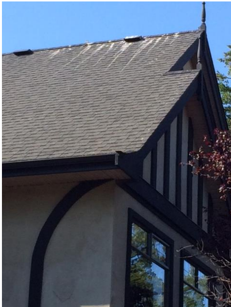
Appendix Figure 18. A close-up of the feces build-up on the peak. Note the proximity of the feces to the air shaft.
