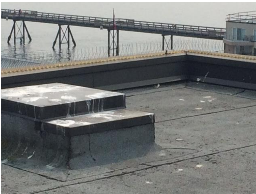
Appendix Figure 30. Despite the installation of the spikes, gulls still manage to perch and defecate upon small infrastructures on flat roofs.
