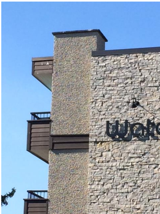
Appendix Figure 16. Note the proximity of the gull feces to the living quarters of the residents.
